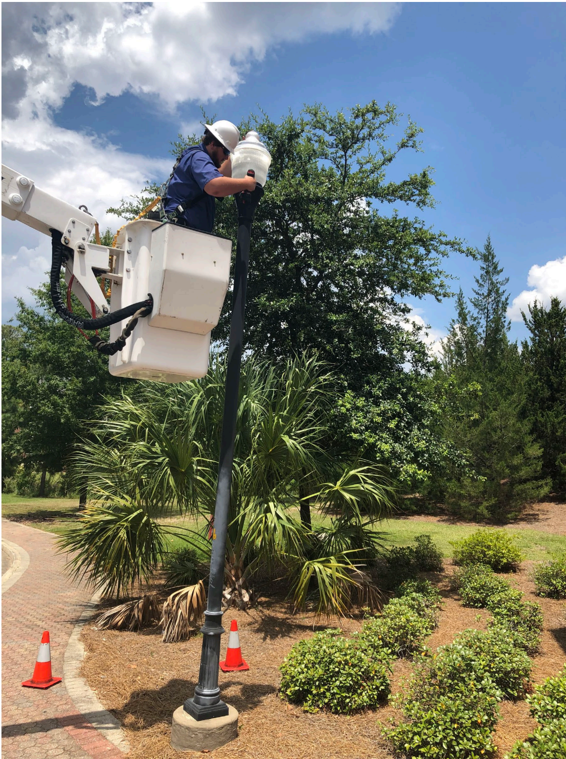
Electrical Shop employee Garrett Bland participating with install of Pedestrian LED upgrade
