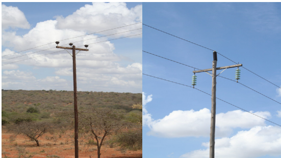
Figure 1a & b. 1a (on the left) shows the typical “T-structure” which poses an electrocution risk to birds perching on the cross arm. 1b shows the “inverted T” pole structure which is safer for perching birds since the outer conductors are suspended below the cross arm out of reach of birds.
