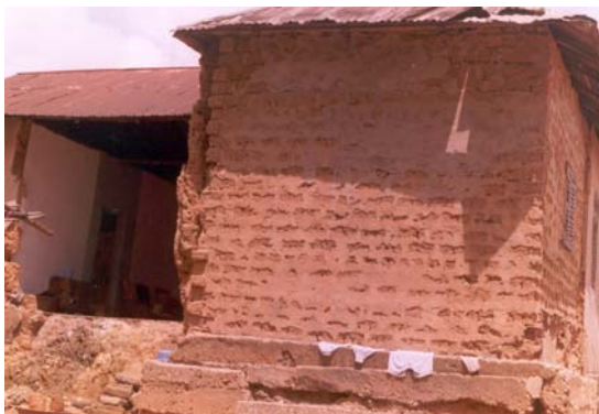
Fig. 1 A Landcrete House with Distressed Foundation
