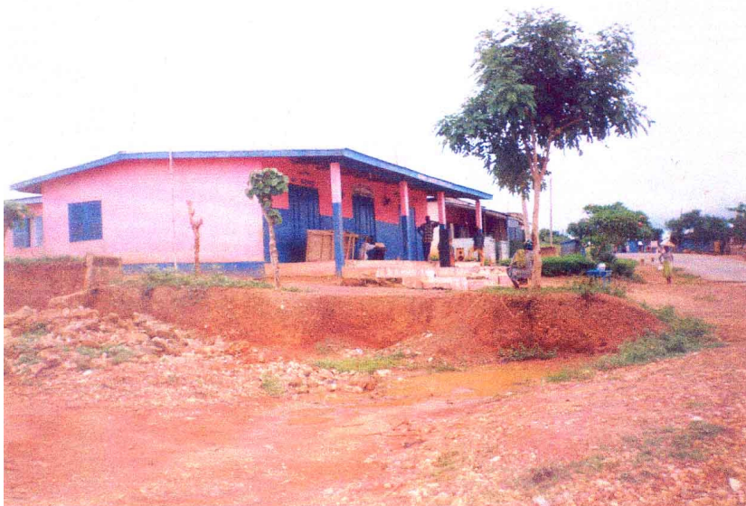
Plate 2: A section of the Boadua to Akwatia road degraded including nearby building
