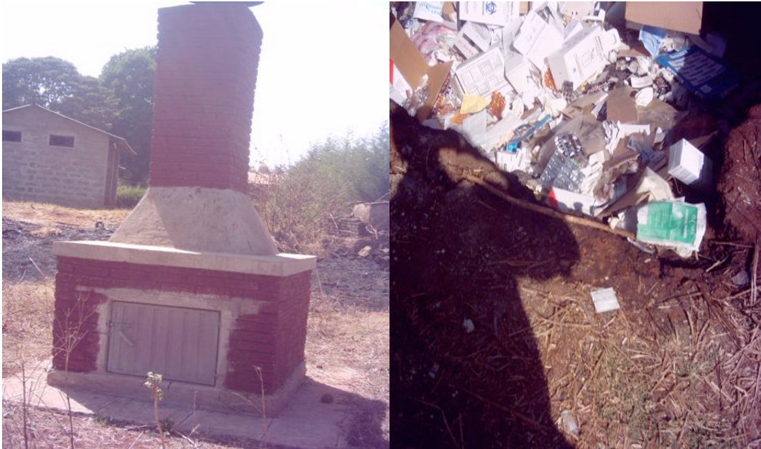
Figure 1: Newly constructed incinerator for HCW disposal and mixed disposal of HCW with open pit in study health centers.
