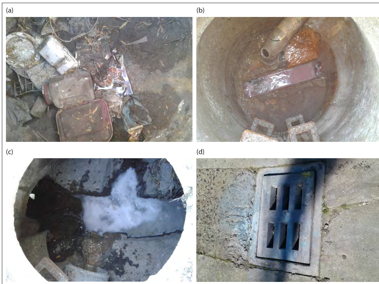
Figure 17. Photos of illegal discharges in manholes on Alternator Avenue: (a) Manhole 5ALT filled with stones; (b) Manhole 11ALT with pinkish discharge; (c) Manhole 7ALT with white soapy foam discharge; (d) stormwater inlet with stain
