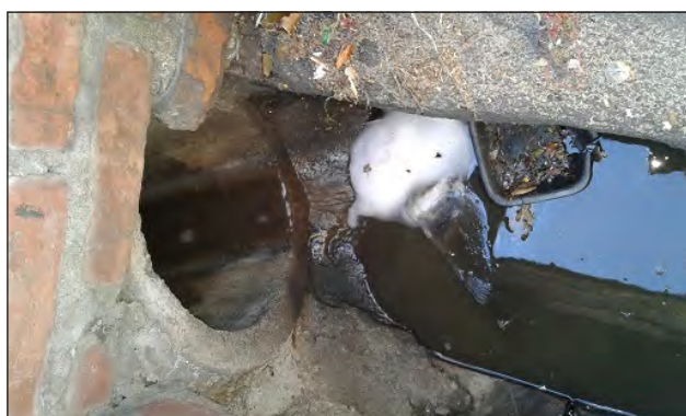
Figure 12. Carwash effluent discharging into Manhole 19MON
