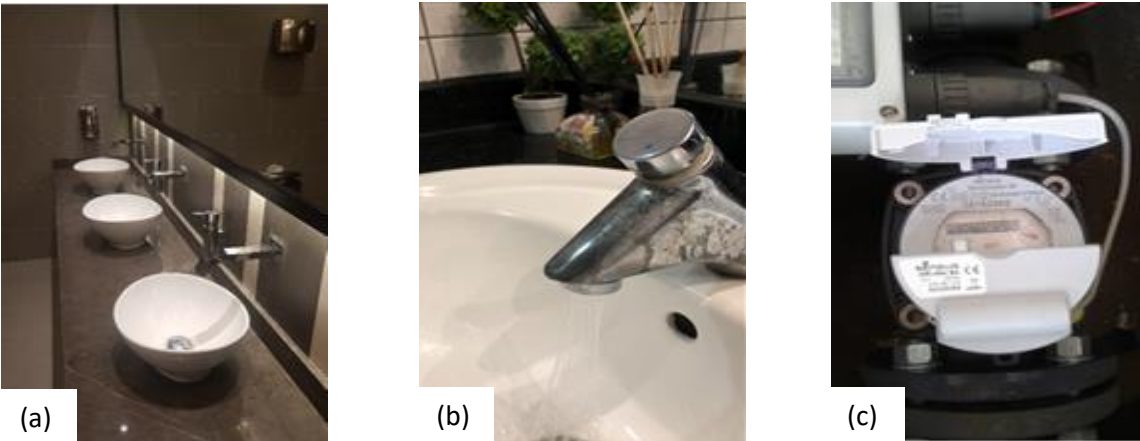
Figure 2: (a & b) Faucet aerators: Automatic & low flow nozzle faucets installed in all academic buildings including on-campus mosques and (c) Smart water meter to manage water usage
