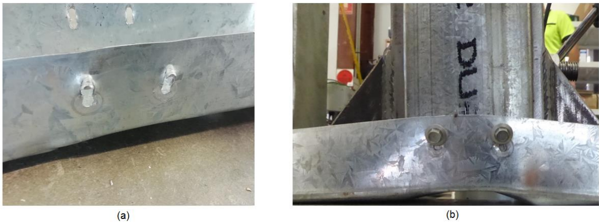
Figure 3.14. Failure modes of the track: a) Screw bearing, b) Track buckling
