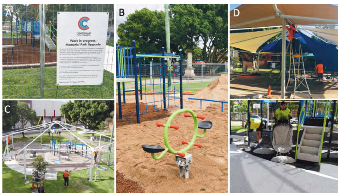
FIGURE 27: Main stages of the playground transformation in September and October 2020. (A) Closing the playground to the public. (B) Ground works to remove old surface materials and new subgrade. (C) Installation of the steel frame for shade sails. (D) Mounting shade sails into the frame. (E) Pouring the new surface material.
