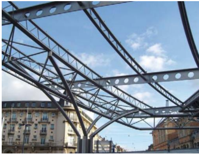
(a) Structural stainless steel at Gent Sint Pieters railway station in Belgium. Photo: Patrick Lints [1]
