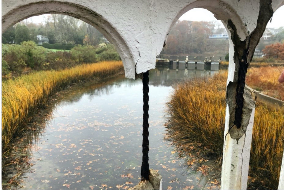
Figure 8: Damaged balusters showing exposed twisted rebar, November 2020.
