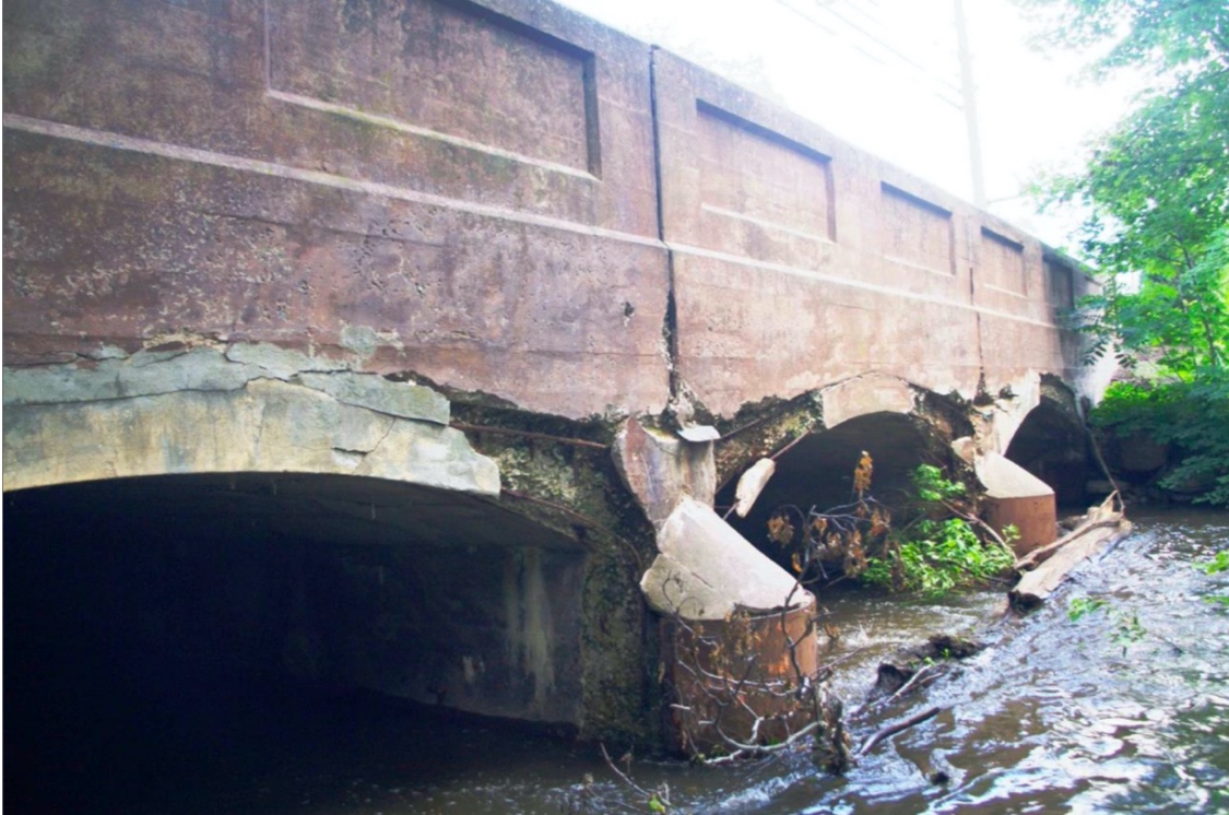
Figure 6.7: Damage to the western spandrel wall, 2018. Source: CT DOT Update of 1991 Connecticut History Bridge Inventory, Bridge 3651.
