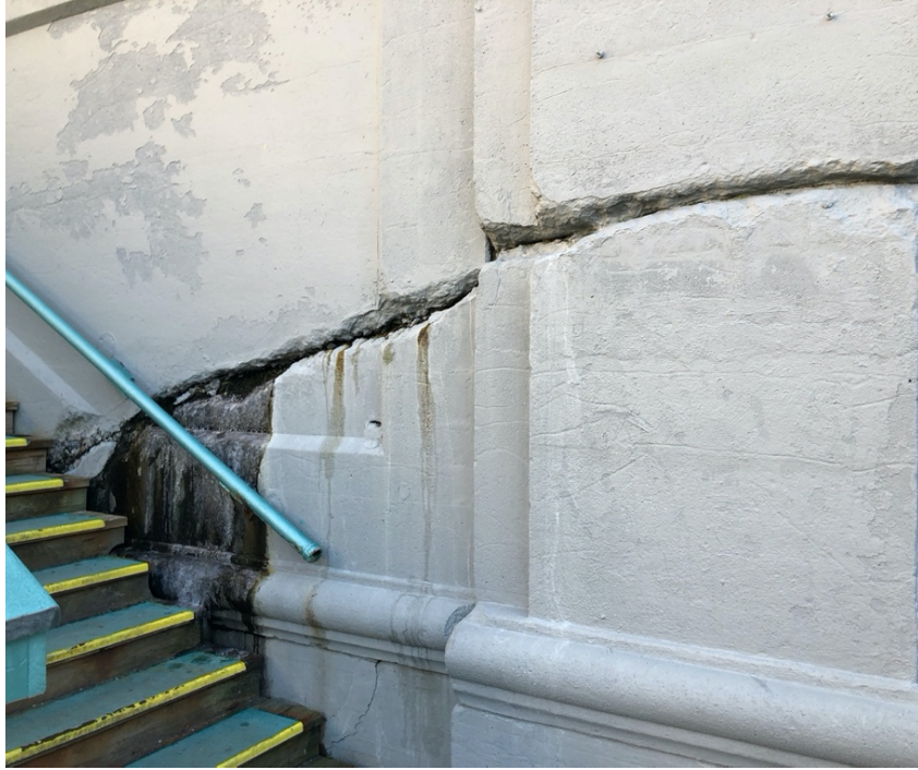
Figure 7.11: Cracks in the northern side wall of the east abutment, January 2021.
