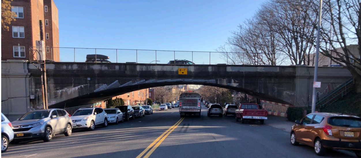
Figure 7.1: The north side of the Seeley Street Bridge over Prospect Ave, January 2021.
