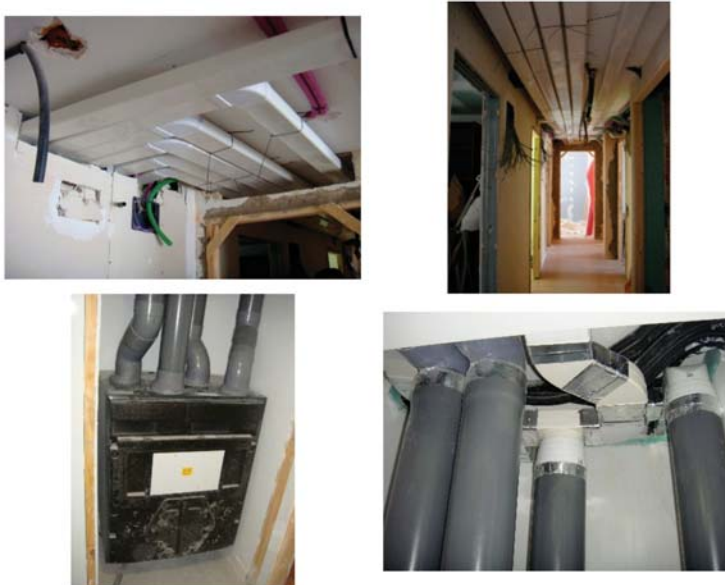
Figure 15. Double duct ventilation facility installed in the dwelling.
