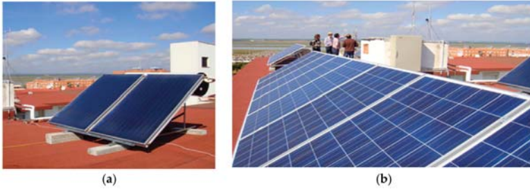
Figure 16. (a) Flat solar thermal collectors; (b) Photovoltaic panel facility.
