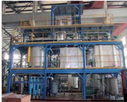
Figure 8. First industrial scale SCWO plant in China [71].
