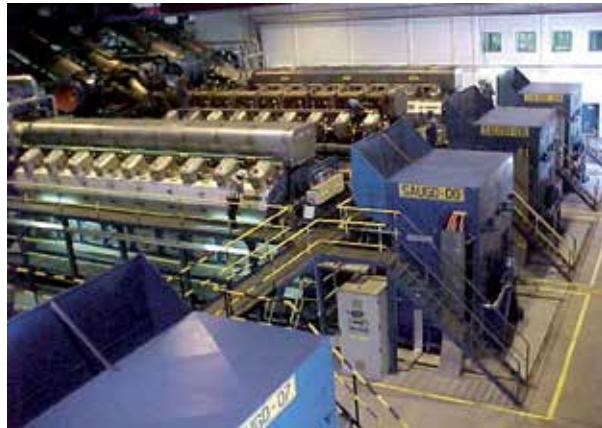
Figure 2. Diesel generating units, at Santana Thermoelectric Power Plant.
