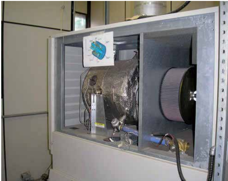
Figure 7. Capstone microturbine in the laboratory at UNIFEI.
