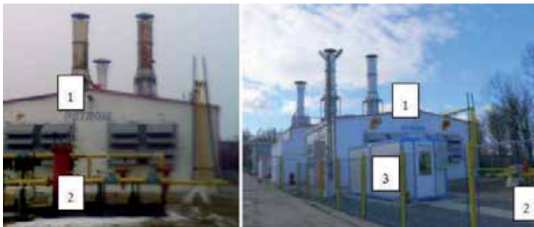
Figure 4. Control – measurement station for natural gas at 2xST 18 – Suplacu de Barcau plant (left) with booster (right) 1 – cogeneration power plant; 2 – control – measurement station; 3 – booster
