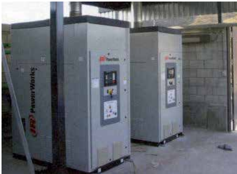
Figure 3. Ingersoll-Rand Power Works™ installed on the Jamacha Landfill - United States.
