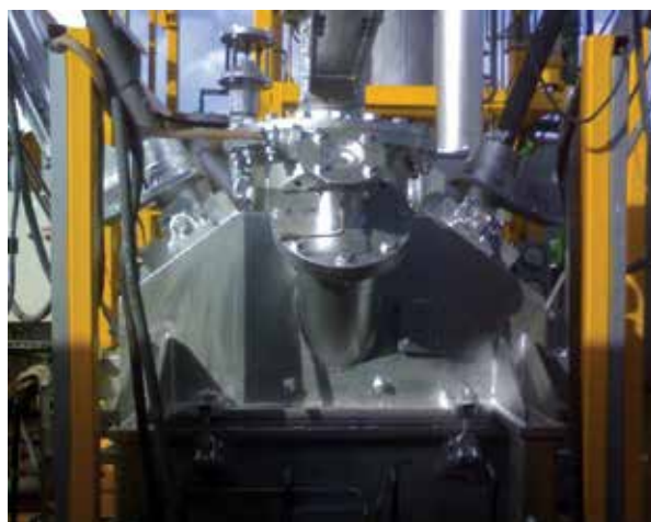
Photo 7. Gasification / vitrification furnace
