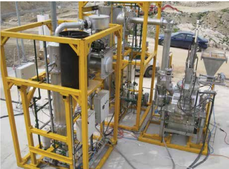
Photo 5. Another general view of the demonstration gasification / vitrification unit
