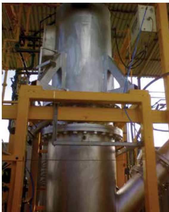
Photo 17. Secondary Combustion Chamber
