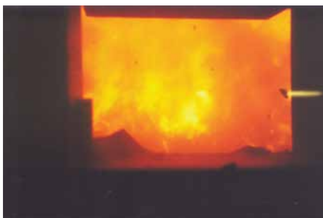
Fig. 3. Inside of an incineration chamber in Valorsul's incinerator (S. João da Talha, Loures, Portugal).
