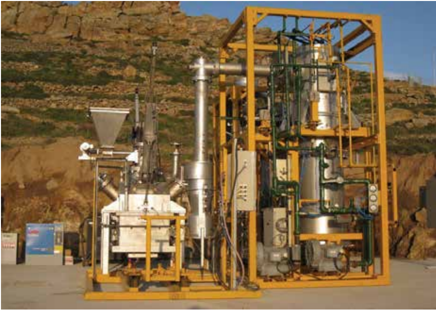
Photo 4. General view of the demonstration gasification / vitrification unit
