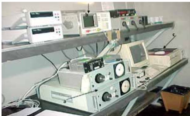
Fig. 4. Internal view of the control room (courtesy of IFI/DCTA, Brazil).
