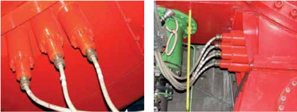
Fig. 15. Signal cable glands
