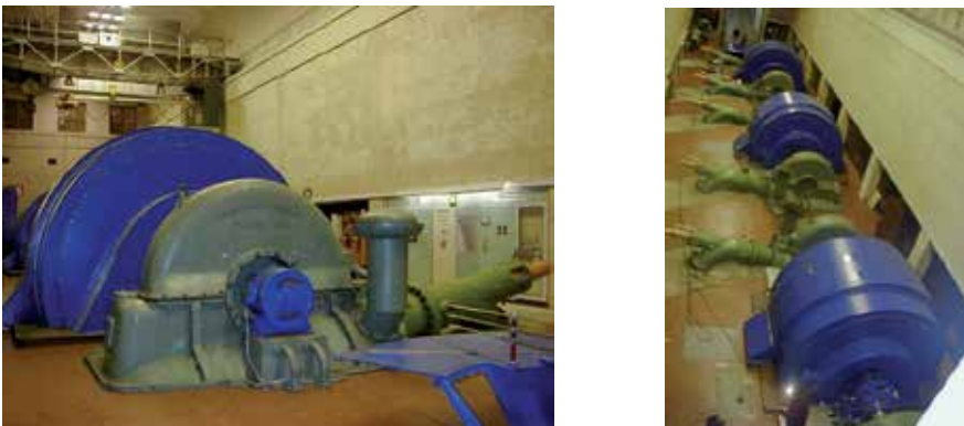
Fig. 1. Hydro-generators in hydro power plant Vinodol - 35MVA each
