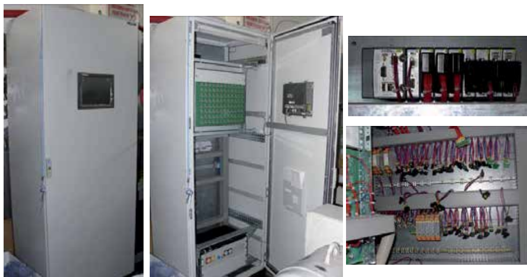
Fig. 13. Measurement cabinet for measurement systems installed on all three generators in hydro power plant Vinodol
