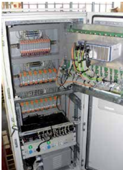
Fig. 16. Measurement cabinet with NICDAQ9188 data acquisition system
