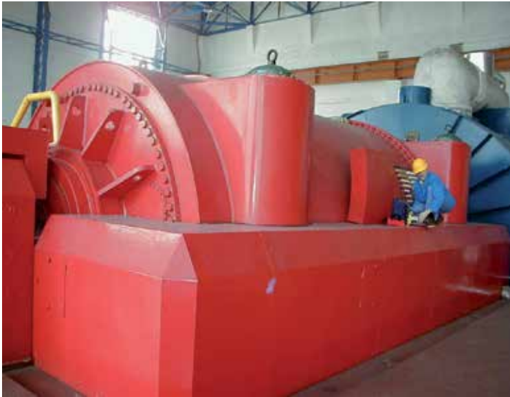
Fig. 14. Turbo-generator 250 MVA in Plomin 2 thermo power plant
