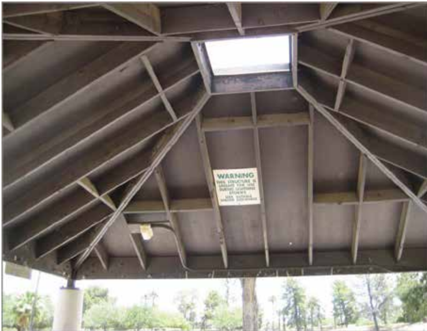
Figure 13. Lightning-unsafe small structure. Note sign recommending a safe place elsewhere rather than staying at this location (©R. Holle).
