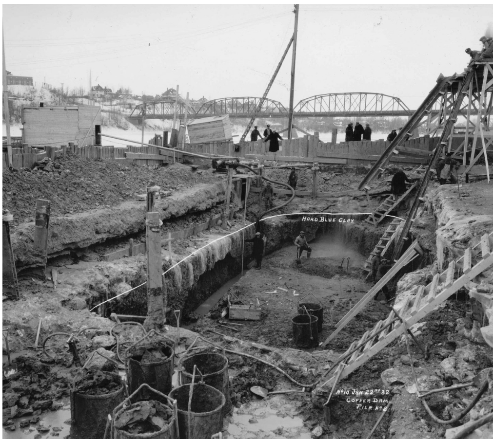
Figure 5. The construction of Saskatoon's Broadway Bridge, 1932. Relief workers in a cofferdam lay the foundations for the bridge's second pier, using hand shovels to carve through the dirt and hard blue clay. In the upper left is the pump house, where river water was pumped out of the cofferdam. City of Saskatoon Archives, 1104-003-006.
