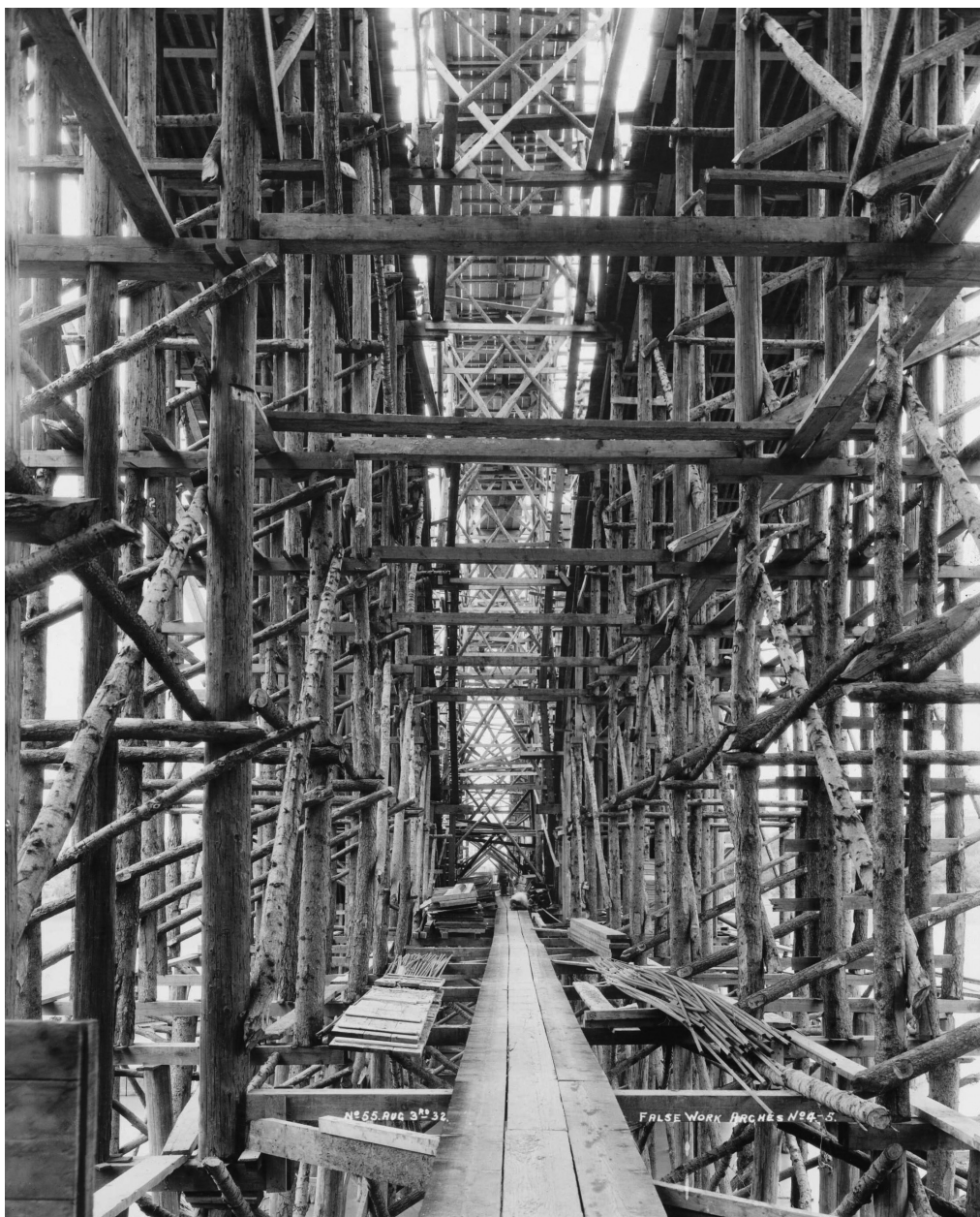
Figure 6. The elaborate falsework of the Broadway Bridge's arches, 1932. Workers mixed cement on the riverbank of the South Saskatchewan River, loaded it into wheelbarrows, and then manoeuvred the wheelbarrows along the narrow wooden trundle before dumping it into the pier forms below. City of Saskatoon Archives, 1104-003-045..
