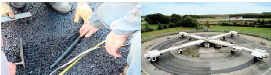
Figure 4. Installation of fiber optic cable at IFSTTAR accelerated pavement testing facility—pavement fatigue carousel (figures are reproduced from Chapeleau et al. [40]).
