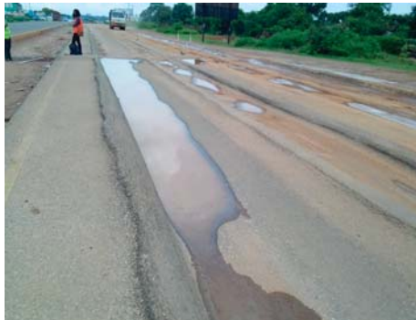
Figure 9. Extent of rutting (Kitwe-Chingola).
