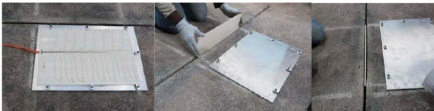
Figure 5. Instrumented plate installation at the Federal Aviation Administration (FAA) National Airport Pavement Test Facility (NAPTF) in Atlantic City, New Jersey, USA (figures are reproduced from Garg et al. [45]).
