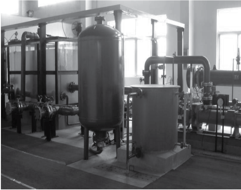
Fig. 6. Photograph 2 of the test system (containment sump strainers)
