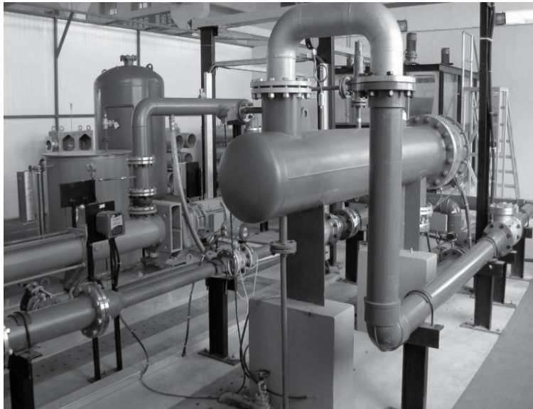
Fig. 5. Photograph 1 of the test system (containment sump strainers)
