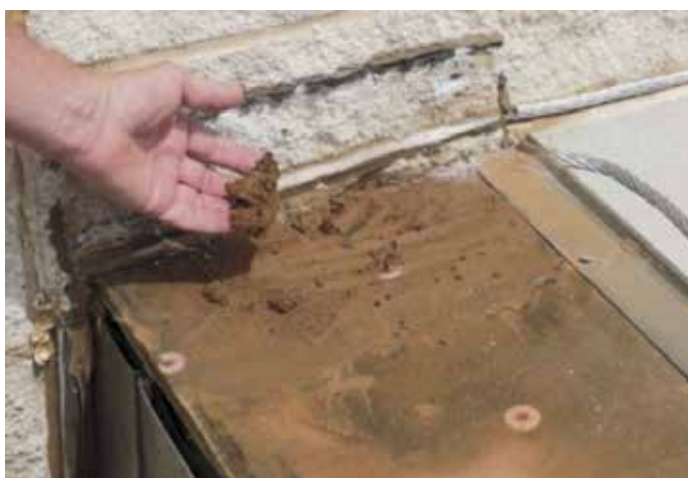
Fig. 13. Infiltration of dirt and moisture under parapet cap.
