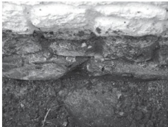
Fig. 2. The copper-coated base flashing at the applied masonry veneer wall terminated below grade and therefore did not allow for the water to drain.
