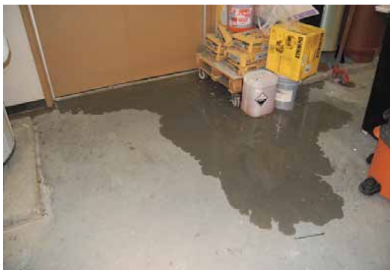
Fig. 7. A flawed detail at the base of the building compounded the threat to the building posed by standing water.
