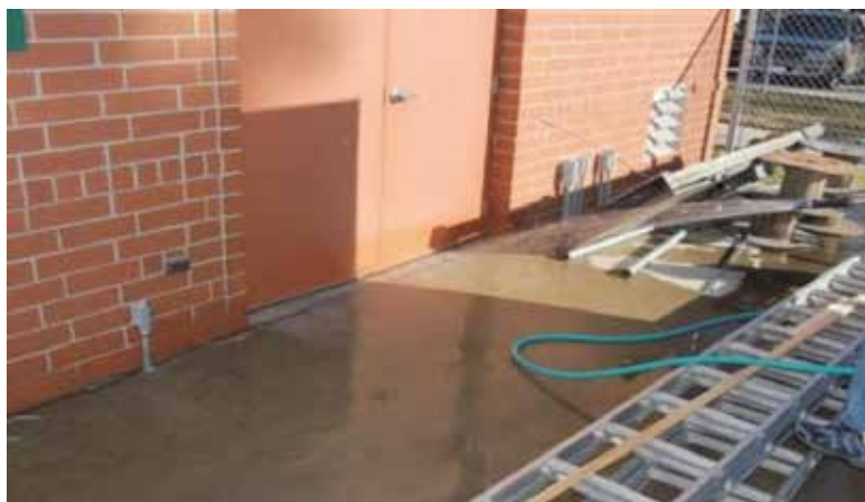
Fig. 6. Site drainage violated code and held water against the building.
