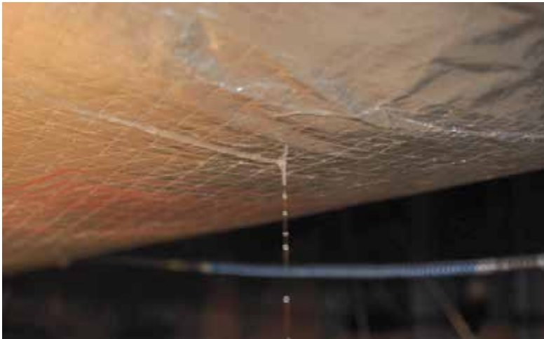
Fig. 10. Water running out of insulation.
