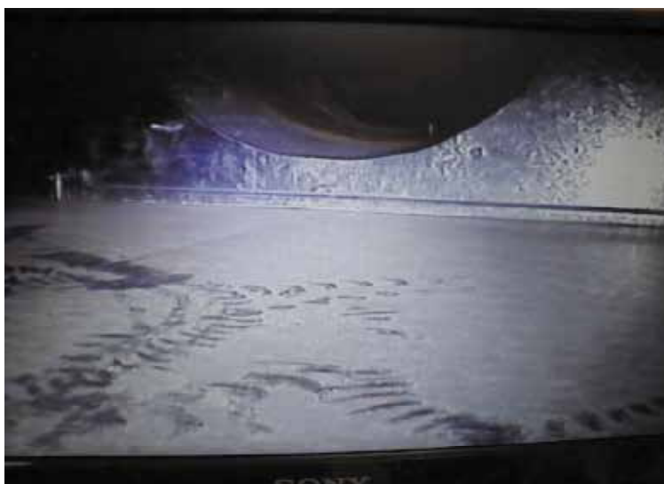
Fig. 16. Tracks of robotic camera in the dust of the HVAC ductwork.
