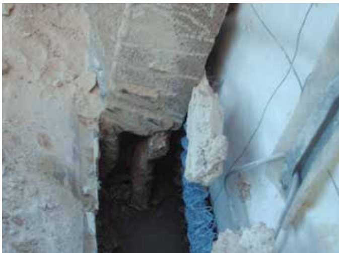
Fig. 12. Water standing inside wall cavity.
