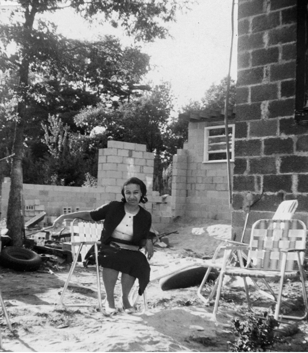
FIG. 1.3 A 1960s view of the building site with my neater masonry to the left and a family friend, Joanne Jackson (Spann), seated in the foreground.
