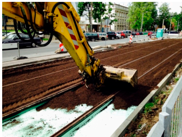
Figure 8. Reconstruction of a tram line—laying a lawn, Rakowiecka Street, Warsaw. Photo: J. Łukaszkiwicz, V 2015.
