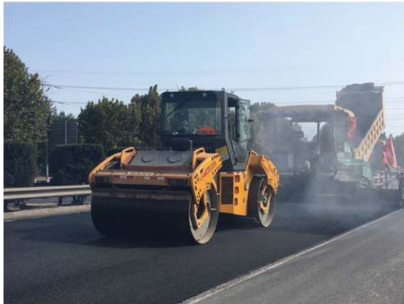
Figure 5. Mechanical equipment used for asphalt paving and compaction: pitch paver and road roller.
