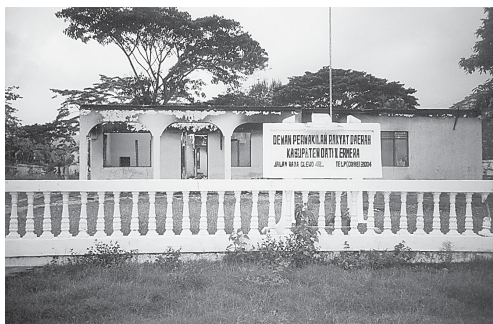
District Parliament Building (Dewan Perwakilan Rakyat Daerah) in Gleno, Ermera, destroyed in September 1999
