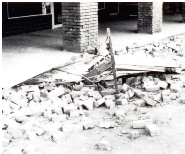
Figure 7. Failure of a commercial sign in the 1979 Imperial Valley, California earthquake (FEMA E-74, 2012).
