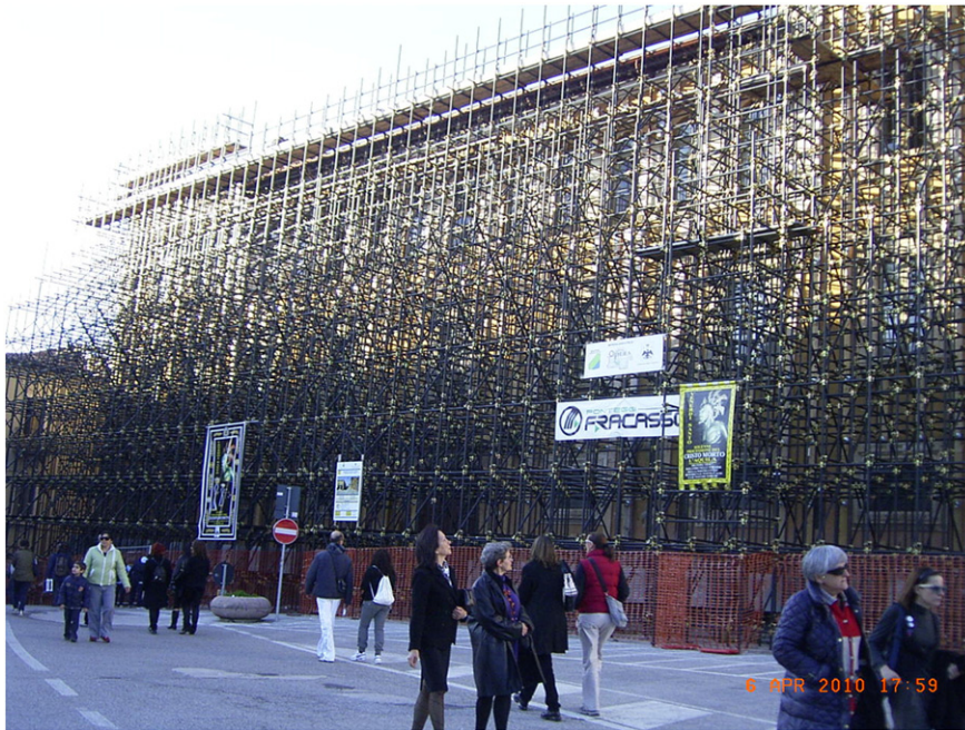
Fig. 7. Cordoned off area in the former business center of L'Aquila city (Italy). April 6th, 2010 (one year after the earthquake).
