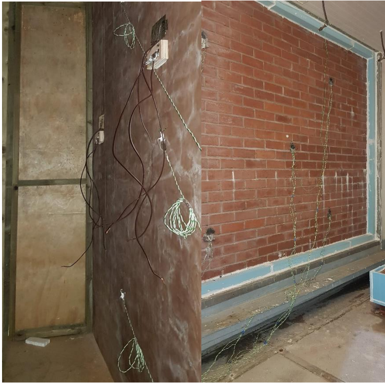
Figure 3-3 Salt Deposits on both Plaster Face and Brickwork
