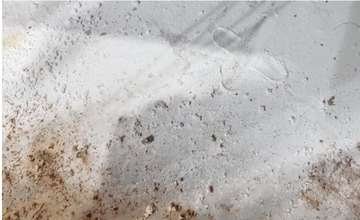
Figure 3-1 Salt Deposit Leached from Bricks
