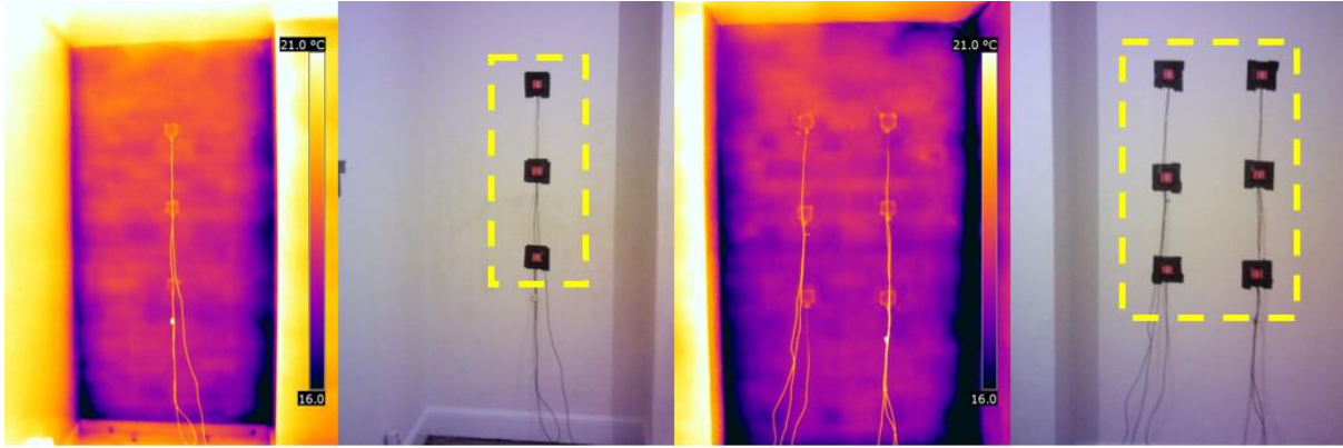
Figure 3-3 Thermogram showing surface temperature variation across the baseline external wall of Test House C (left) and the HFP grid arrays (within the yellow rectangles) used to derive the in situ U-value
