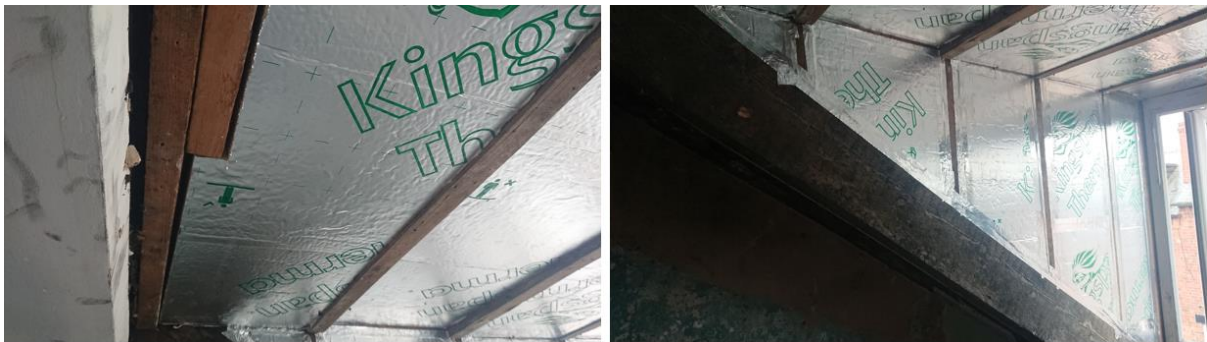
Figure 7-5 Conventional RiR retrofit work. Gaps evident around edges of insulation boards prior filling to taping between upper dormer beam and adjacent dormer ceiling joist (left) and recessed insulation boards on dormer ceiling (right)
