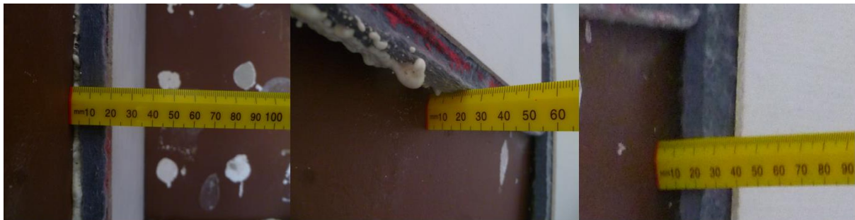
Figure 3-12 Foam adhesive dabs applied to TIWI 2 indicating variation in the airspace thickness behind the insulation boards of between 5 mm to 15 mm
