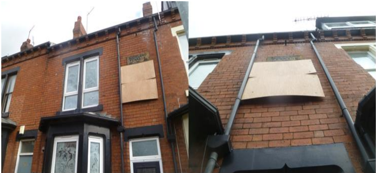
Figure 3-4 External plywood shielding mounted on the west façade of House B to prevent direct solar radiation impinging of the wall surface at the location of the HFP grid array
