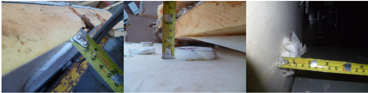
Figure 3-11 Plasterboard adhesive dabs applied to IWI and TIWI 1 indicating variation in the airspace thickness behind the insulation boards of between 5 mm to 25 mm
