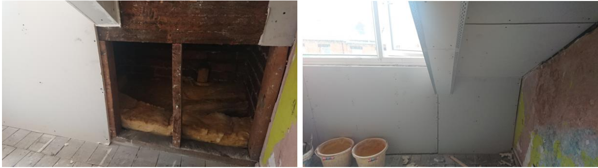
Figure 7-4 TIWI over-boarded RiR retrofit work. Insulation being installed in the residual loft space behind the knee wall (left). Small gaps evident between TIWI boards (right)
