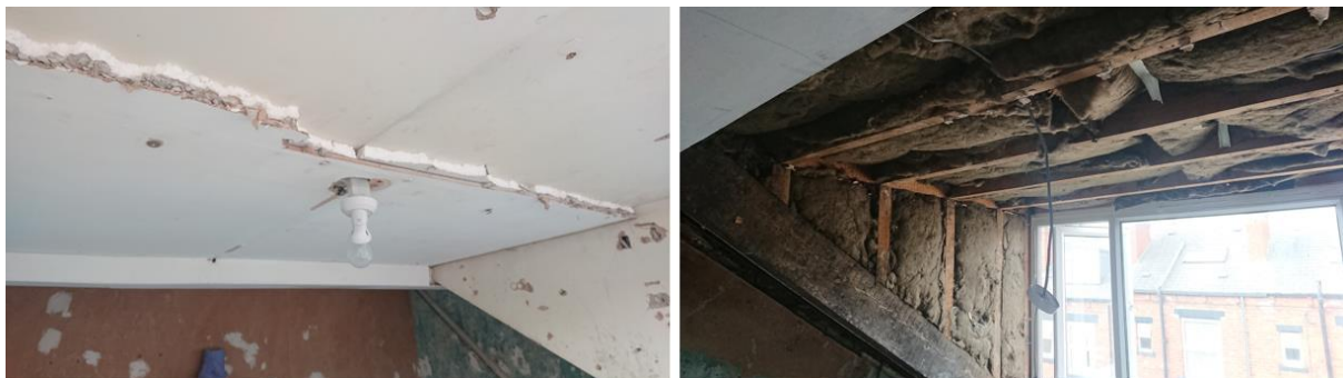
Figure 7-2 Pre-existing EPS plasterboard being removed from the ceilings of House D prior to handover (left). Mineral wool found in dormer of conventional retrofit RiR following baseline tests
