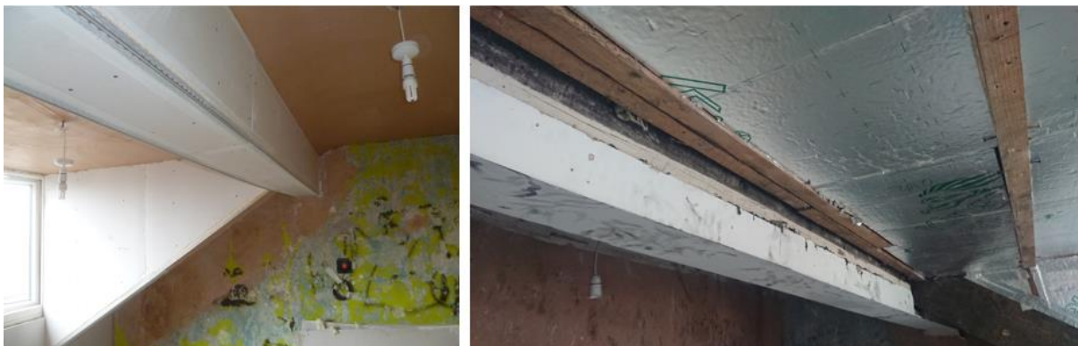
Figure 7-6 Upper dormer beam and dormer trimmer rafter for each RiR. TIWI was used to overboard these timbers (left) whereas timbers were left untreated in conventional RiR retrofit (right). Channel between the upper-dormer beam and adjacent dormer ceiling joist (right)
