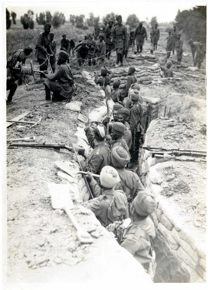
Figure 9. Indian infantry dig trenches at Fauquissart, France. Trenches became the defining physical feature of the warfare adopted on the Western Front, but by the Indian Army Corps Headquarters' own admission, the expeditionary force arrived ill-equipped to participate in such warfare. 55
