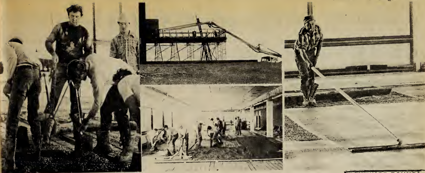
Work on the third floor of C/D's A building continues. In the left picture, workmen are shown spreading the concrete that comes through a hose from the mixer outside of the building. Center (top) — The structure that supports the base. Center (bottom) — Workers lay the cement for floors of future classrooms. Far right — A worker puts the finishing touches on a slab of cement. The third floor will supposedly be similar to the second floor. — Photos by Scott Salter.
