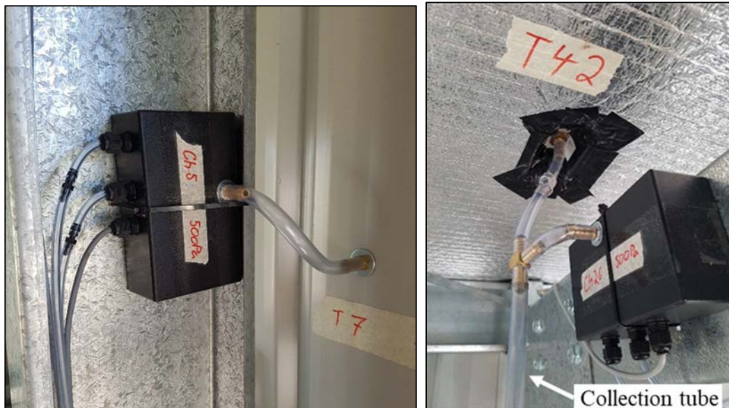
Figure 4.6. Pressure transducers connected to wall tap T7 (left) and roof tap T42 (Right)
