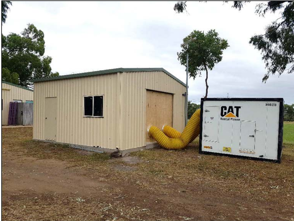
Figure 4.11. Air Handler Unit and flexible ducting attached to the JCU-ASIS via the plywood barrier
