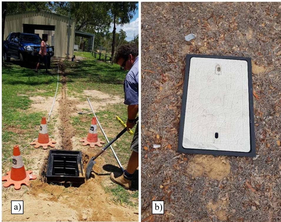
Figure B.7. JCU-ASIS reference pressure pit (a) Installation of underground tubing/conduit into pit (b) Pit in situ with flat lid flush with ground
