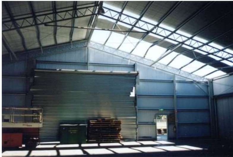
Figure 1.3. Windward roller door failure, generating large positive internal pressures contributing to structural failure - Stehle and Henderson (2001)
