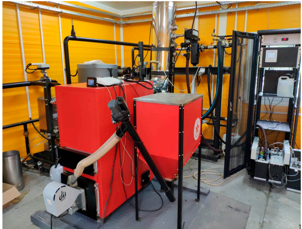
Figure 3. Tested boiler on the testing stand.
