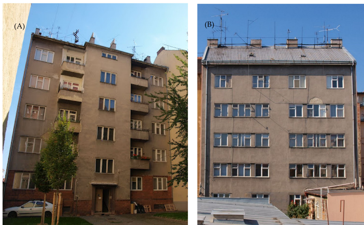
Figure 3. A eastern view (A) and an western view (B) of the neglected and underfinanced residential building before its reconstruction in 2010. Source: Vojtěch Šíp.
