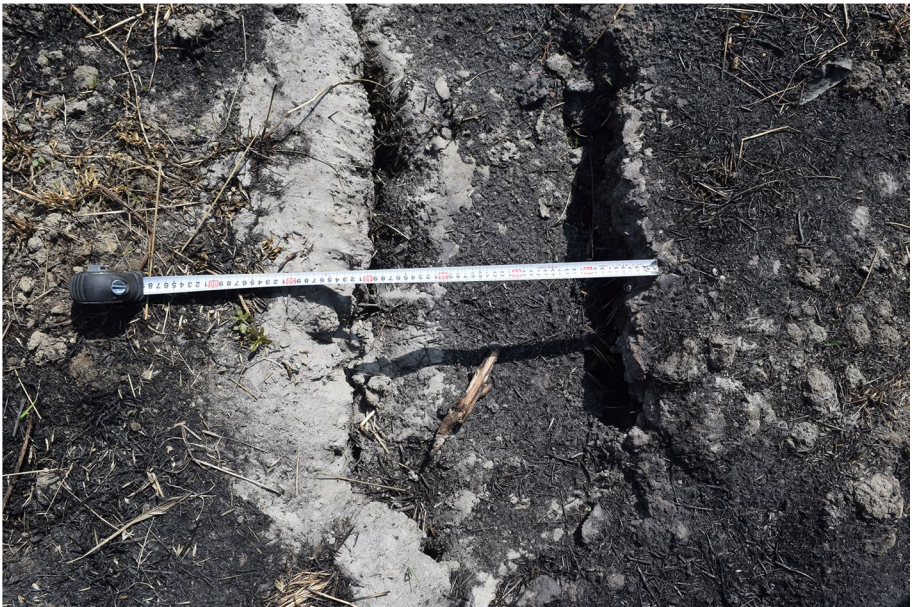
Fig. 11 Liquefaction and sand boiling at Bungmati (Liq. ID 3b in Table 6) [Photo: RM Pokhrel]
