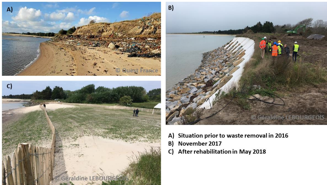
Figure 4. La Samaritaine landfill (a) prior to waste removal in 2016, (b) during waste excavation (November 2017) with erosion being stopped by riprap and a geotextile, (c) the restored site (May 2018). Photography (a) courtesy of Ouest-France archives, (b) and (c) courtesy of Geraldine Lebourgeois/La Presse de la Manche.
