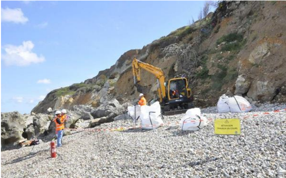
Figure 6. Trial waste removal at the Dollemard landfill (summer 2020). Photograph courtesy of Le Havre council.
