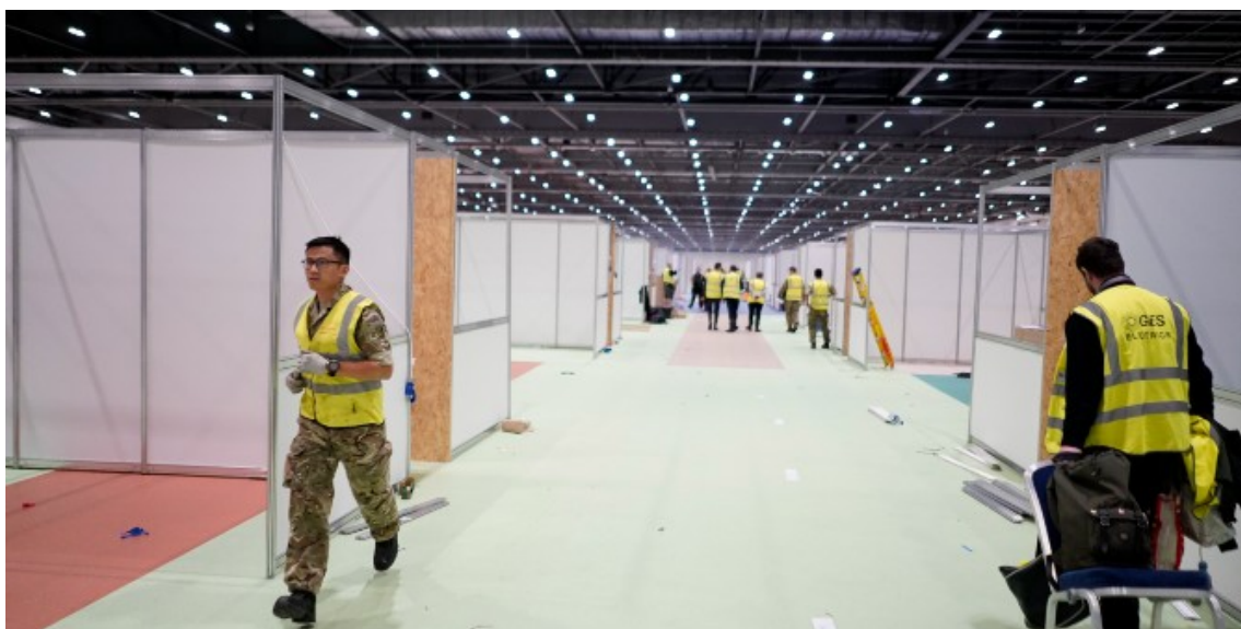
Military staff and contractors build the Nightingale Hospital in east London, March 2020. Photo: Andrew Parsons/ Number 10 via a CC-BY-NC-ND 2.0 licence
