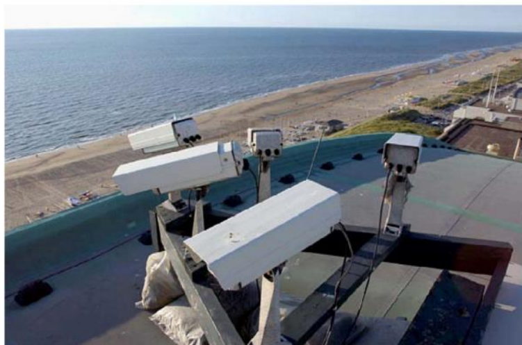
Figure 2.9: The ARGUS camera station at Noordwijk (The Netherlands), installed in 1995. The cameras have fields of view which overlap ensuring the complete beach face is monitored. Image from Holman and Stanley (2007).
