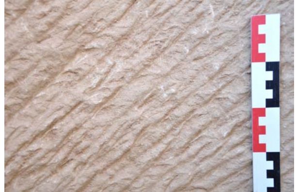
Fig. 64. Inside wall of basin no. 2
