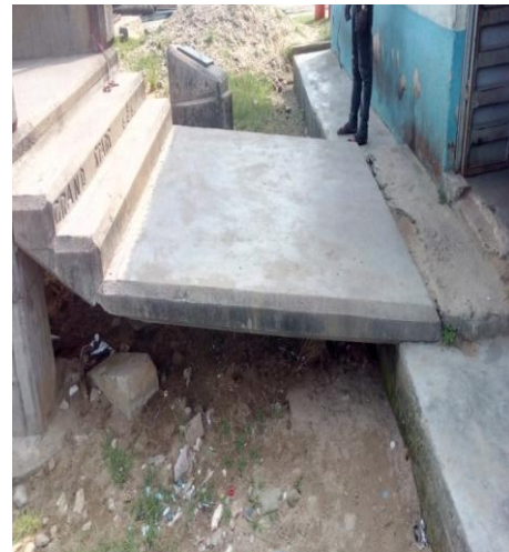
Figure A.10: Image of steps connecting the loading bridge to the terminal building
