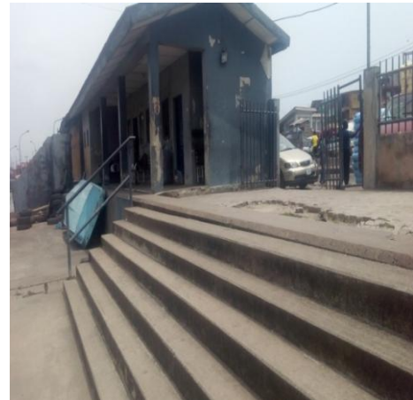
Figure A.16: view of the stairs linking the quay and main entrance to the access road Source: Authors' Field work (2017)
