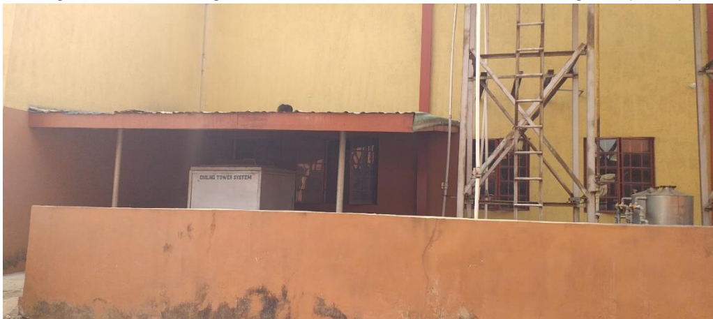
Fig 2.3: Cooling tower system in Federal Institute of Industrial Research
