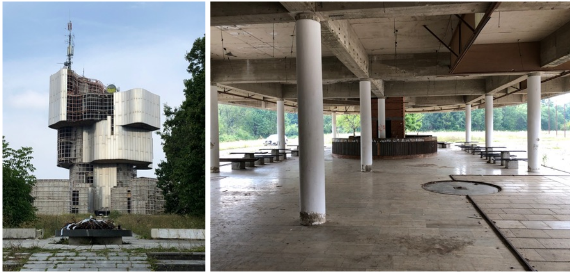
Left: The Monument to the Uprising of the People of Kordun and Banija, showing external stainless steel panels stolen since its abandonment, Petrova Gora, 29 August 2019. Right: The former recreational area at the base of the monument, with picnic tables still intact, Petrova Gora, 29 August 2019.
