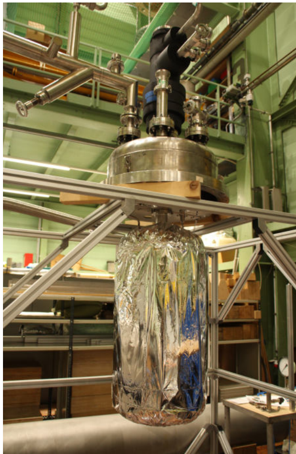
Figure B.1: Photograph of the multi-layer insulated cryogenic vessel exemplary for one blanket of MLI3.
