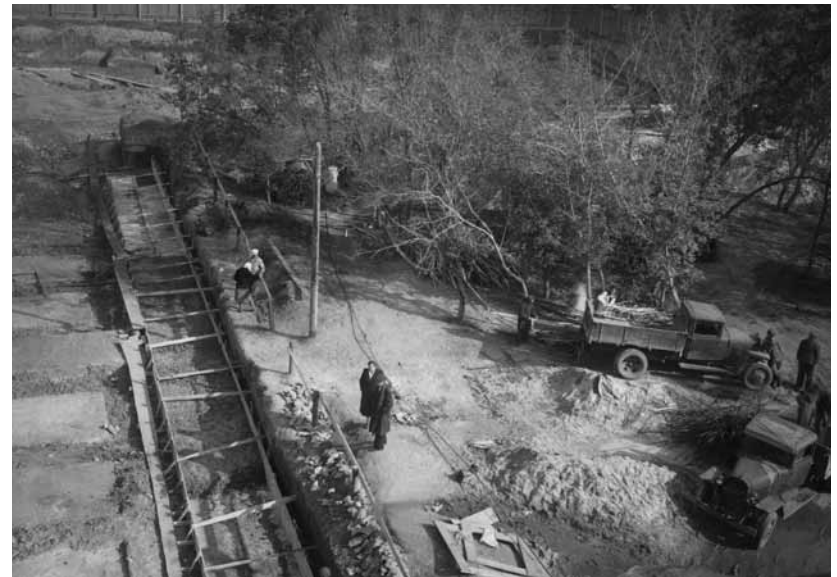
Brigades of librarians and university staff helped builders construct the Saratov University’s new library building. Circa 1950. (Photo, Saratov State University)
