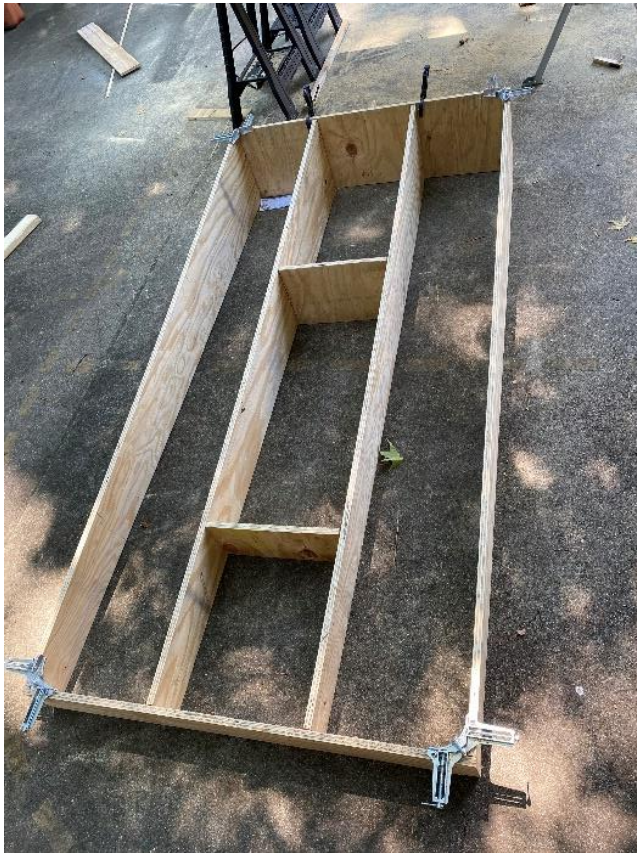
Figure 2. Mound Framework for sloping section. The mound framework was built to Major League Baseball standards and made out of 3/4 inch plywood.
