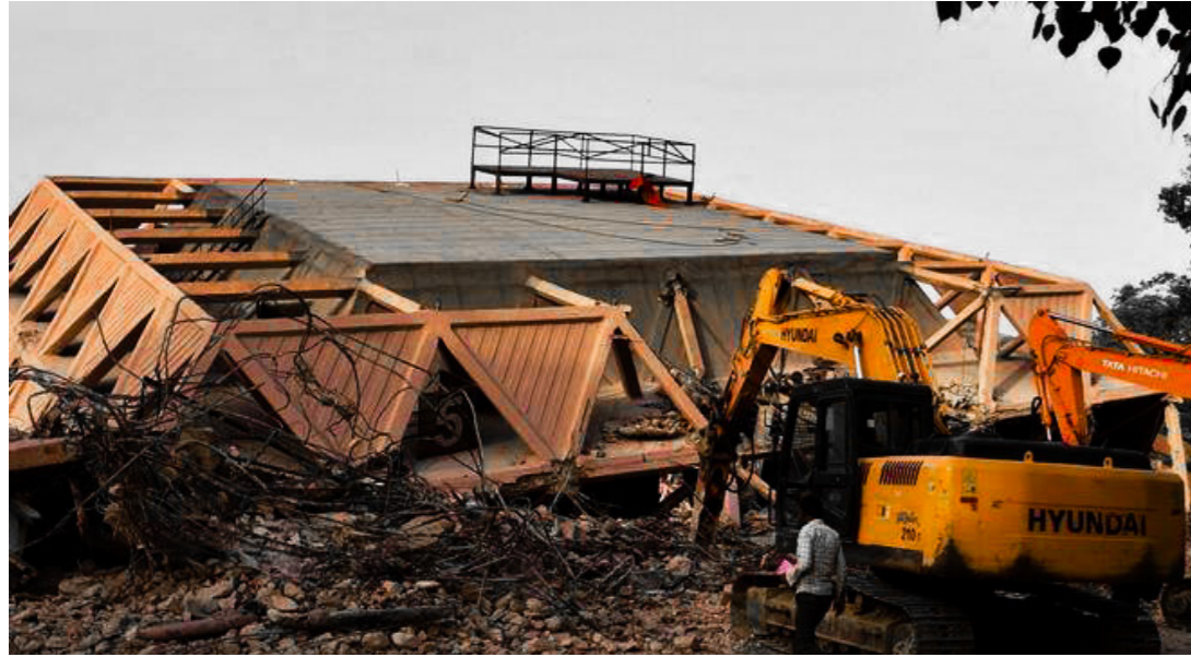
Demolition of Halls of Nation. It was built by Raj Rewal and Mahindra Raj in 1972 and demolished by the New Delhi government in 2017.
