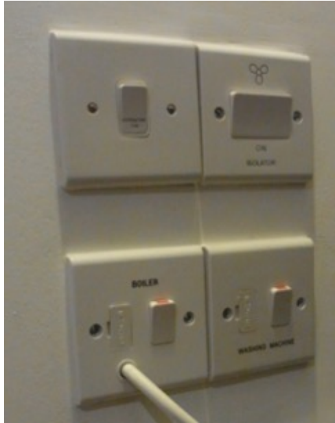
Figure 6.1: Continuous mechanical ventilation isolation switch (top right) amongst other isolation switches in the utility cupboard at CS2.
