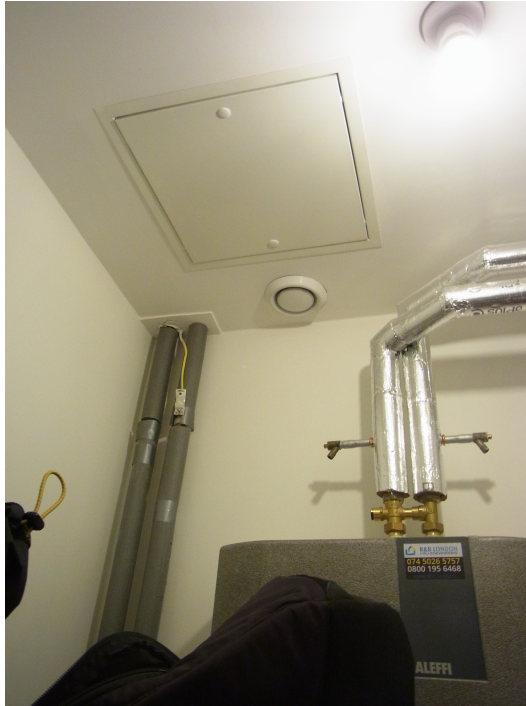
Figure 6.4: Ceiling access panel in the utility cupboard at CS2 for the continuous MEV system and ducts.
