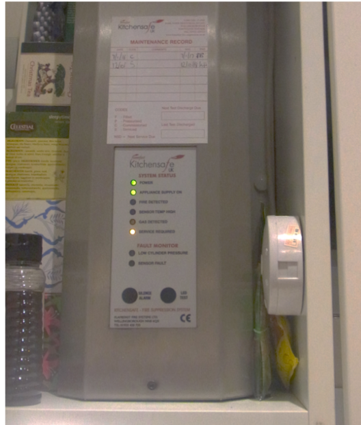
Figure 6.5: Maintenance record sheet and system status indicators on the cooker hood fire suppression system in Flat C.
