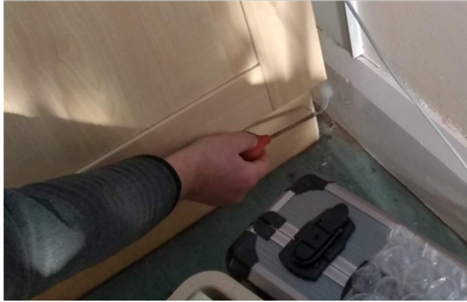
Figure 5.5: Photograph from a smoke survey while UTH was pressurised, showing an air leakage pathway behind the kitchen cupboards.
