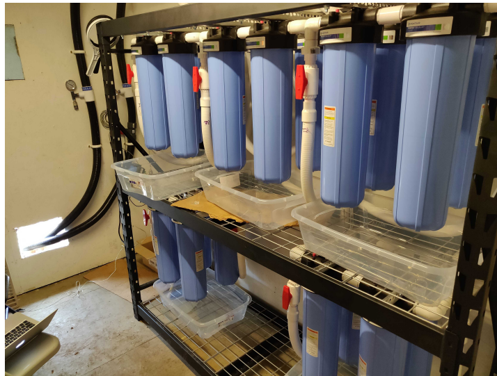
Figure 3.18: Picture of the CHIPS-5 filtration system within one of the shore huts. The pipes to and from the detector can be seen entering and exiting the hut respectively via a gap in the back wall.
