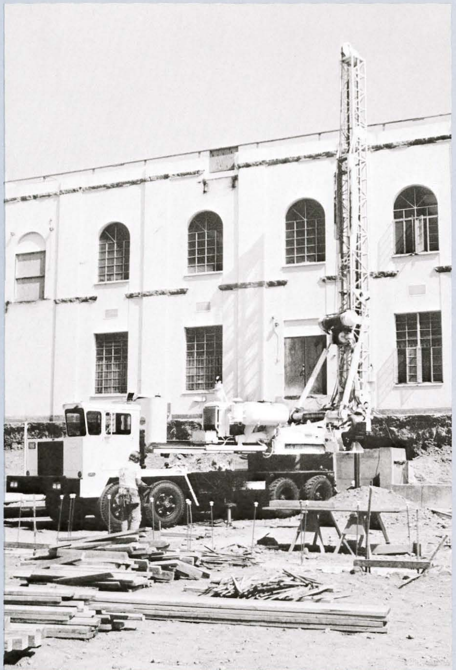
Site preparation began during the summer for construction of a three-story, five-level addition at the back of the Law Library. The addition will more than double the square footage of the facility.
